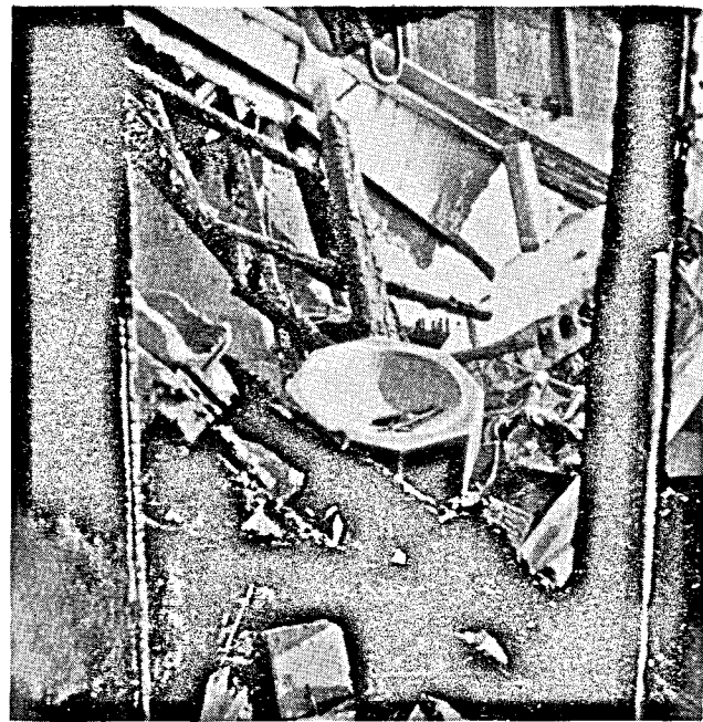
The remains of the Church following the recent fire, which destroyed the church.
