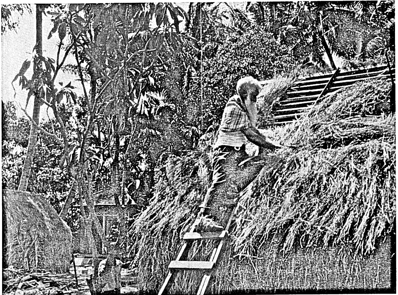
An echo of the past,—construction of a grass house, Hawaiian-style. Photograph by Virgil Biggs.
